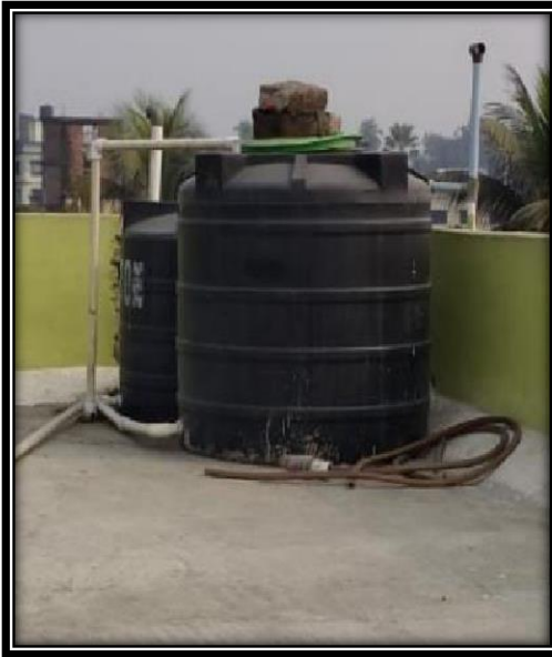
A. Water tanks on roof
