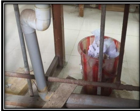
E. Drainage from wash basin
