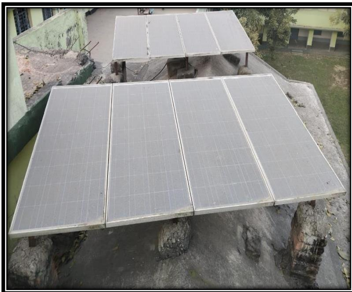
C. Solar panel (top view from rooftop)
