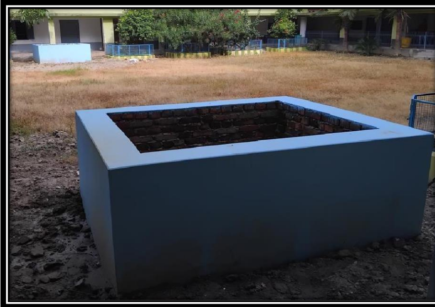
J. Tanks for rain-water harvesting system (storage)
