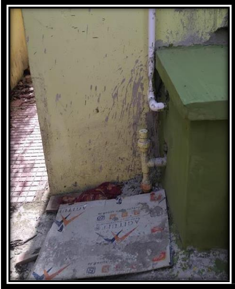
G. Bore-well submersible
