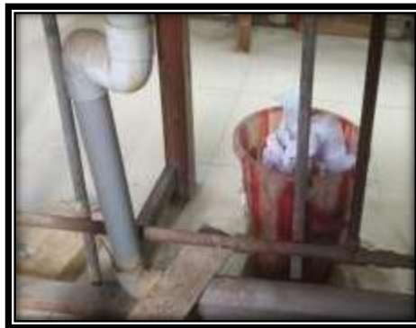
E. Drainage from wash basin
