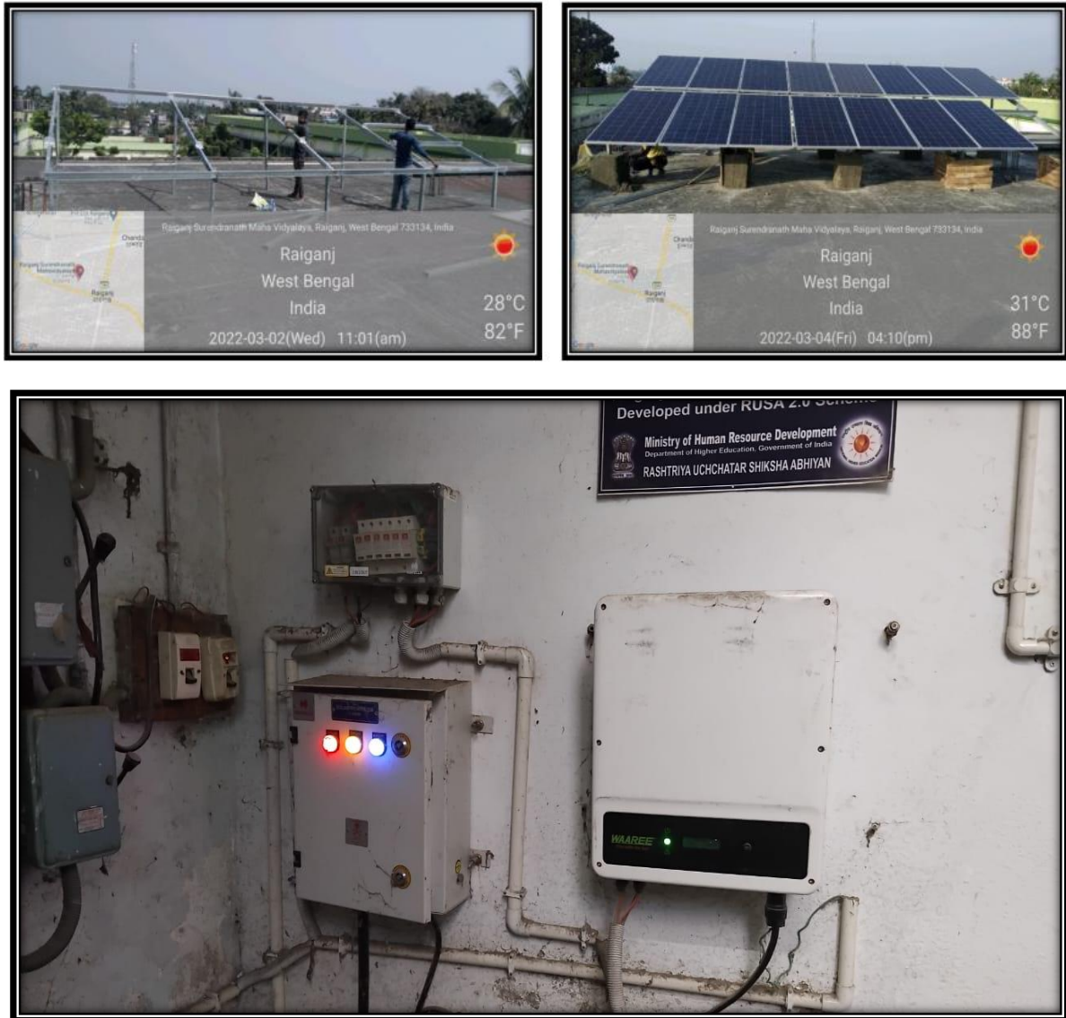
Figure 3: Solar power panels installed at the rooftop of the college building, solar power connection and wheeling to the grid present at the staircase.
