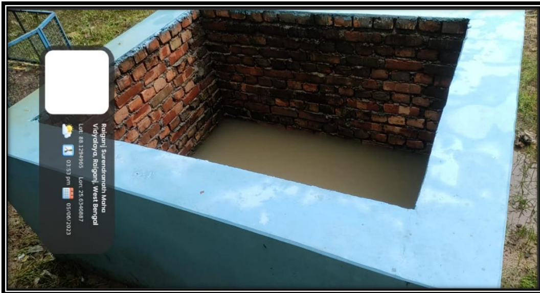
Rain water harvesting (rain water collecting tank)
