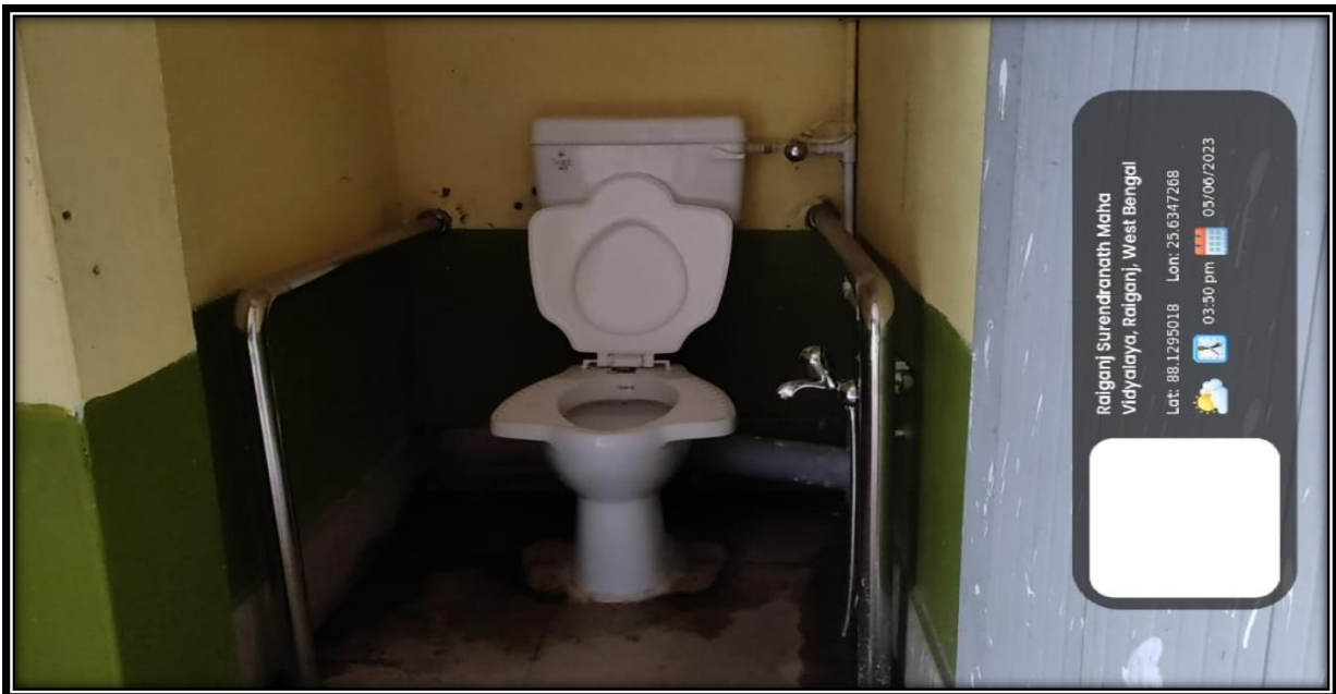
Railing within the toilet for candidates with locomotory challenges
