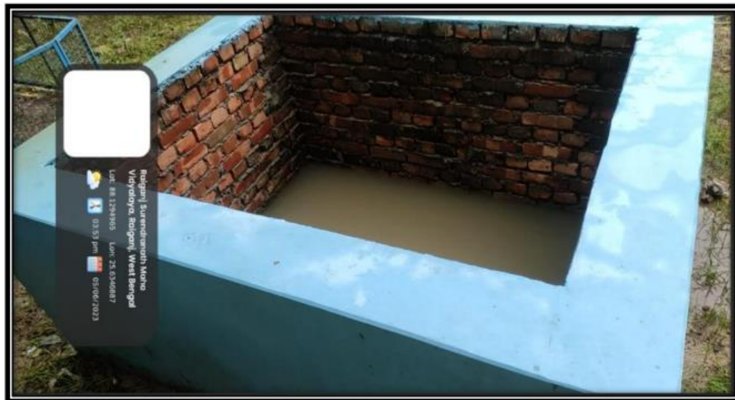
Rain water harvesting (rain water collecting tank)
