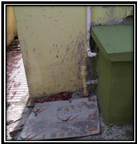
Bore well submersible
