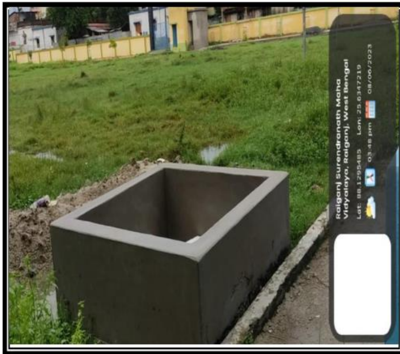
Pit for bio-composting
