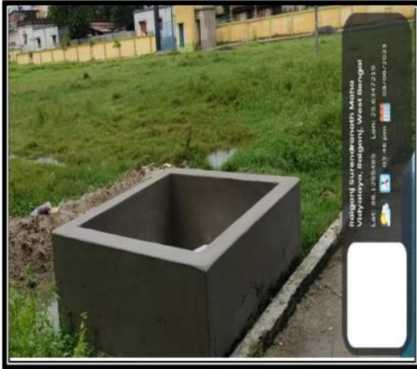
Pit for bio-composting
