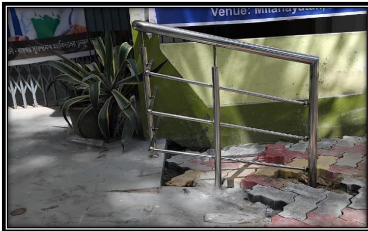
Ramps and railings for persons with locomotor disabilities
